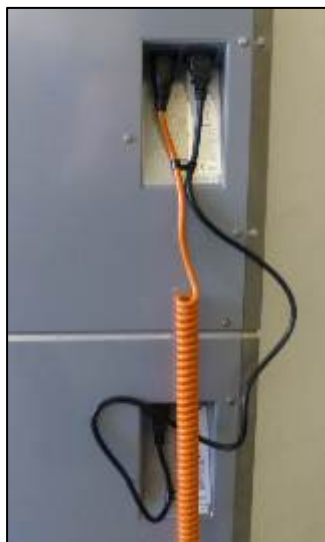
Figure 3b: Mains connection point
